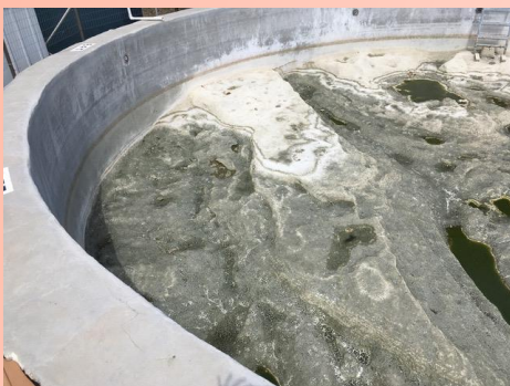
UbarU Pool Leaking (see story on page 5 & 6)
